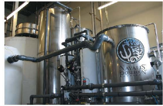
The Navalys Poseidon® Graywater System (back view)
